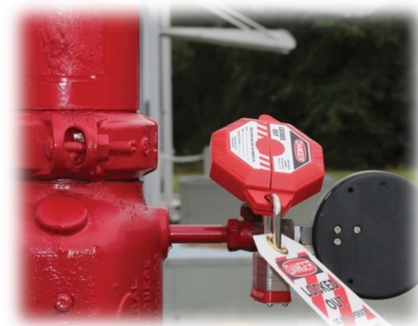
Energy Isolating Device (Valve) with a lockout device (Lockout Device valve cover), lockout, and tagout
